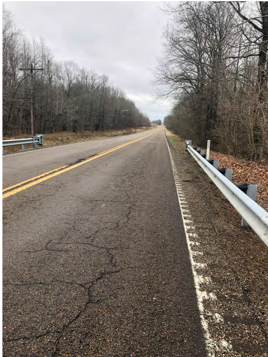
Extensive Pavement Cracking and Rutting Leaving Bridge Eastbound
